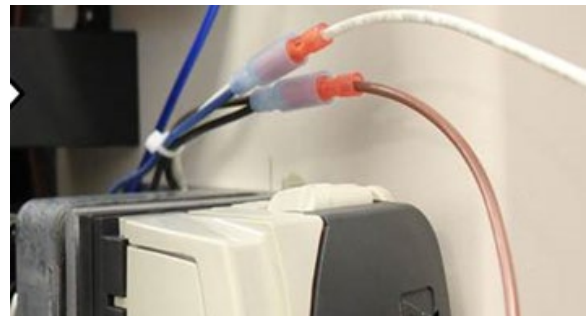
Fig. 3 Disconnecting purge pump wiring
