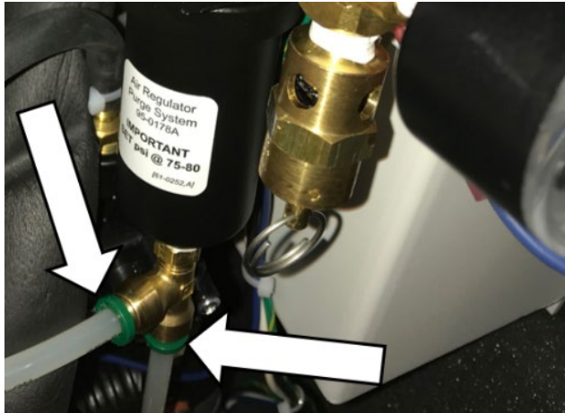
Fig. 11 Connecting tubing to regulator drain
