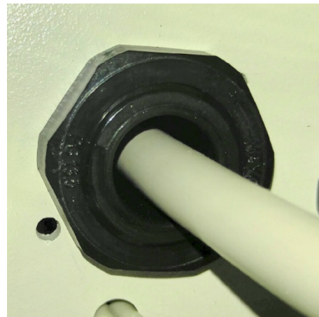
Fig. B2b Inside of Unit
